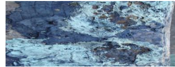
Ineffective tank repairs lead to further deterioration and pitting
