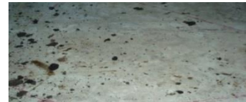
Coating exhibiting spot corrosion
