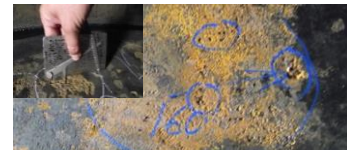
Corrosion and pitting in a tank shell
