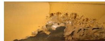
Coating delamination due to insufficient surface preparation or improper coating specification
