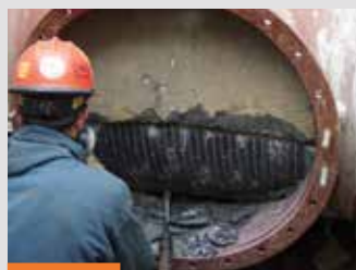
Steel cylinder and concrete wires exposed
