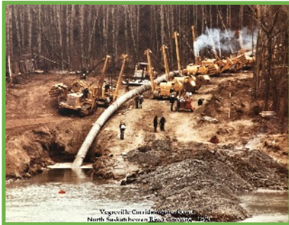
Vegreville Water Board North Saskatchewan River Crossing Submitted by Dale Lefebvre, Town of Vegreville
